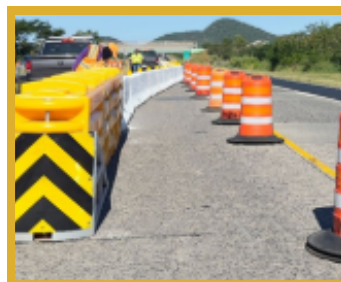
Terminal impact attenuator
