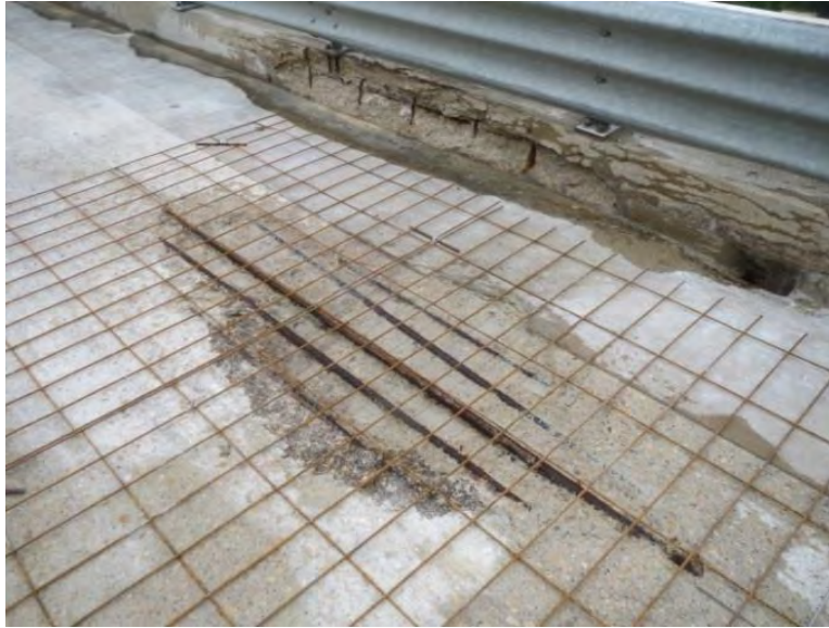
Figure 16. Photo. Distressed region observed on the westbound lane over the pier 1 prior to installing the UHPC overlay.
