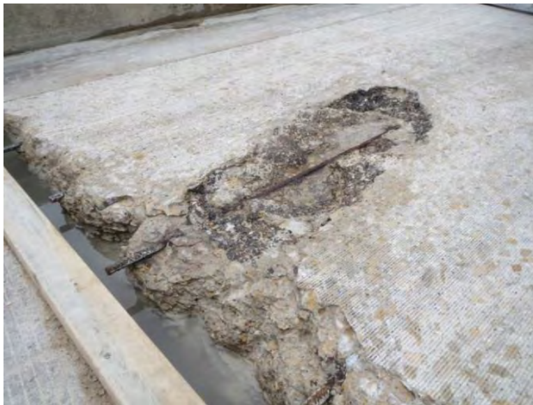
Figure 17. Photo. Distressed region observed on the westbound lane near west abutment prior to installing the UHPC overlay.
