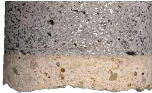
C. UHPC-concrete interface of G3-13 specimen after testing.
