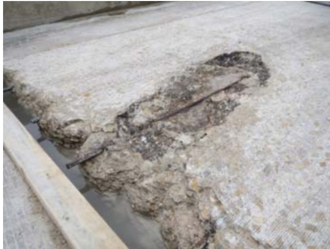
Figure 8. Distressed region on the westbound lane near the western abutment: test region B1. (2)
