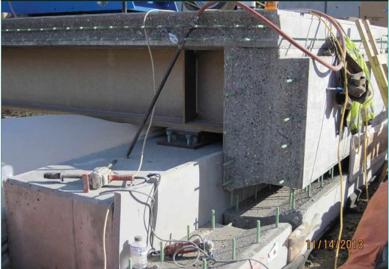
Figure 9. Photo. Semi-integral abutment backwall with vertical and horizontal UHPC connections, I-81 at Preble Road, south of Syracuse, NY.
