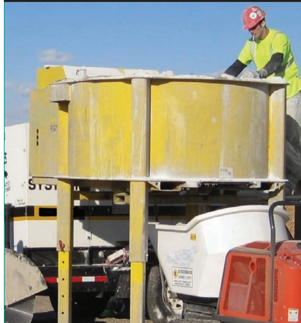
Figure 15. Photo. Portable concrete pan mixer preparing UHPC for placement during the construction of the field-cast connections.
