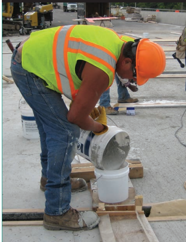
Figure 14. Photo. UHPC placement into a bucket that serves as the overpressure source for a connection. (25)
