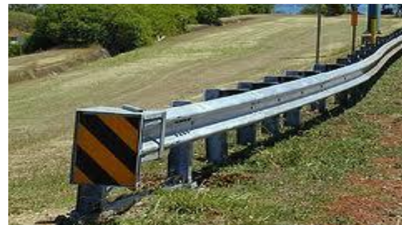
Flared Energy-Absorbing Terminal
