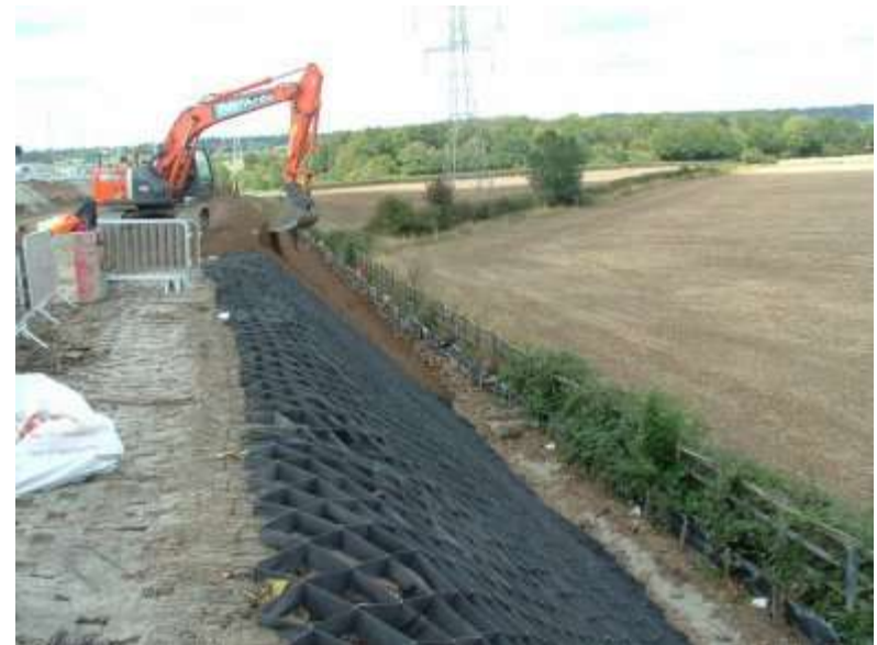
RSS to prevent surface sloughing
