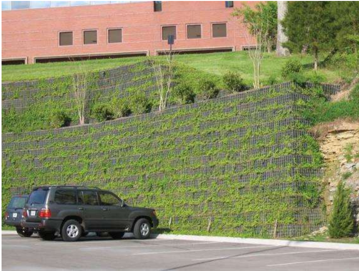
Vegetation growing through the grid structure
