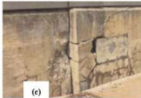
(c) Misalignment of adjacent sections
