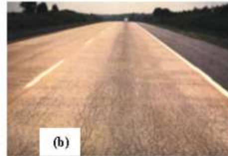
(b) Preferred alignment of cracks
