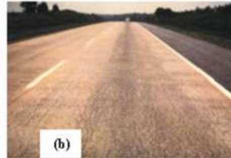
(b) Preferred alignment of cracks
