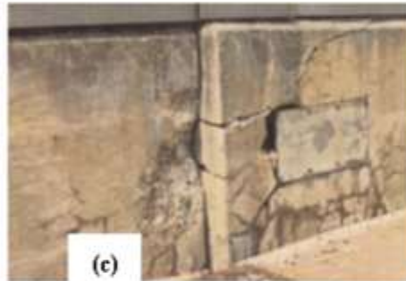
(c) Misalignment of adjacent sections
