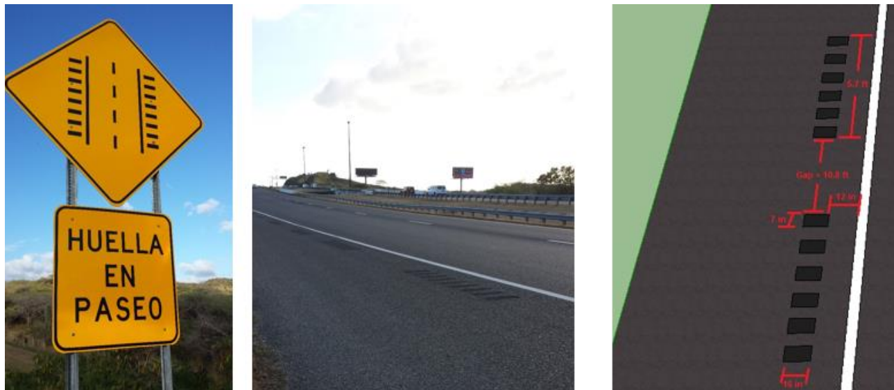
Figure 4: Rumble Strip Sign, Photo of the Rumble Strips on NHS PR-52 Freeway and Dimensions
